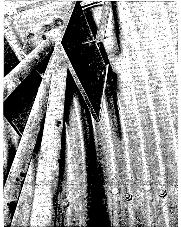
Figure B.2 Scratch deflection gage installed inside conduit.
